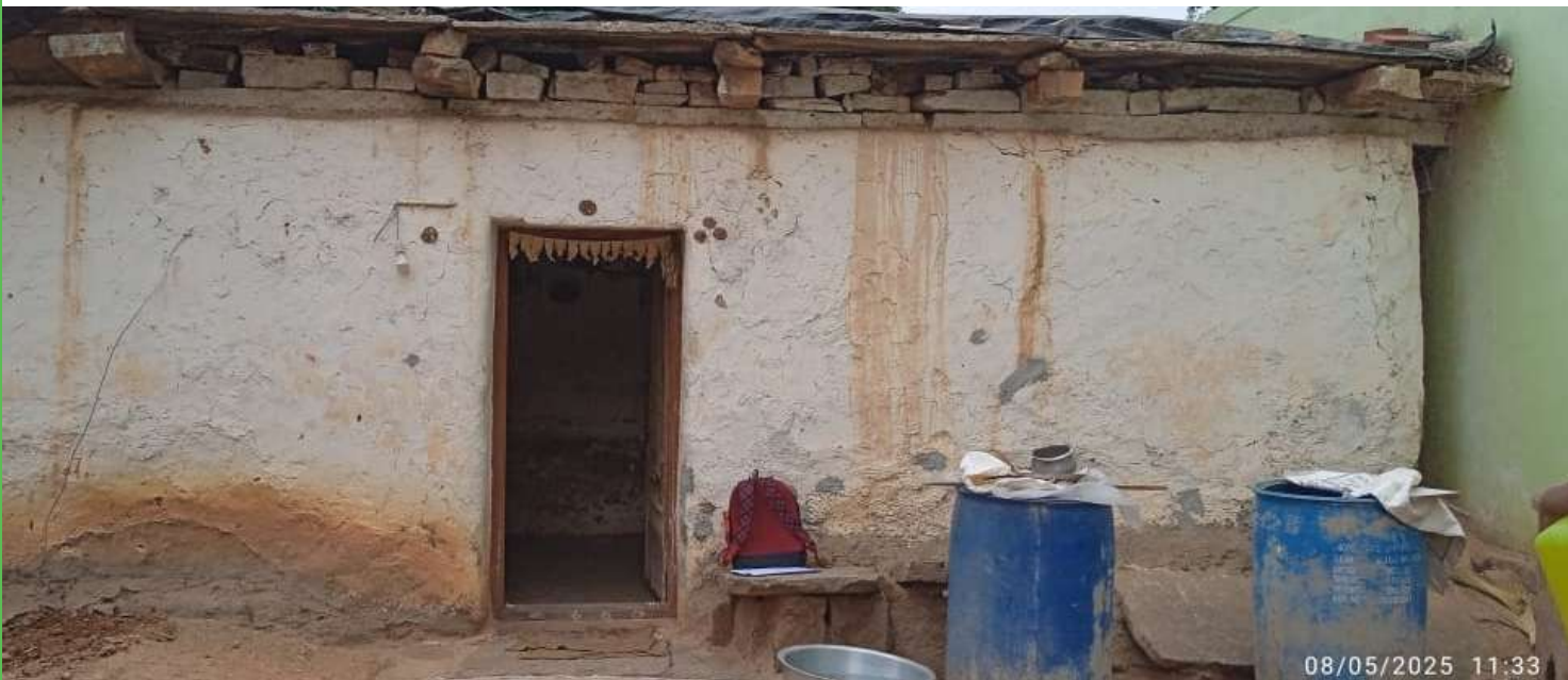
An outdoor view of a rural dwelling with visible signs of heat exposure and temporary roofing adjustments in Udupi, Karnataka.
